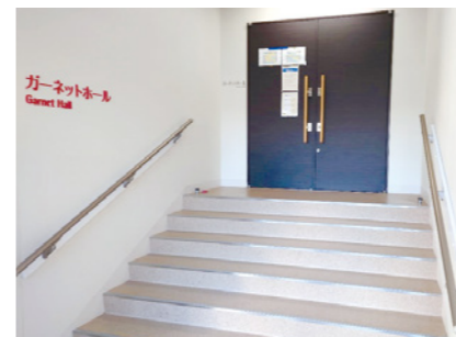
A handrail was installed on the stairs to the hospital's Garnet Hall using a donation from a visitor who tripped on the stairs.
